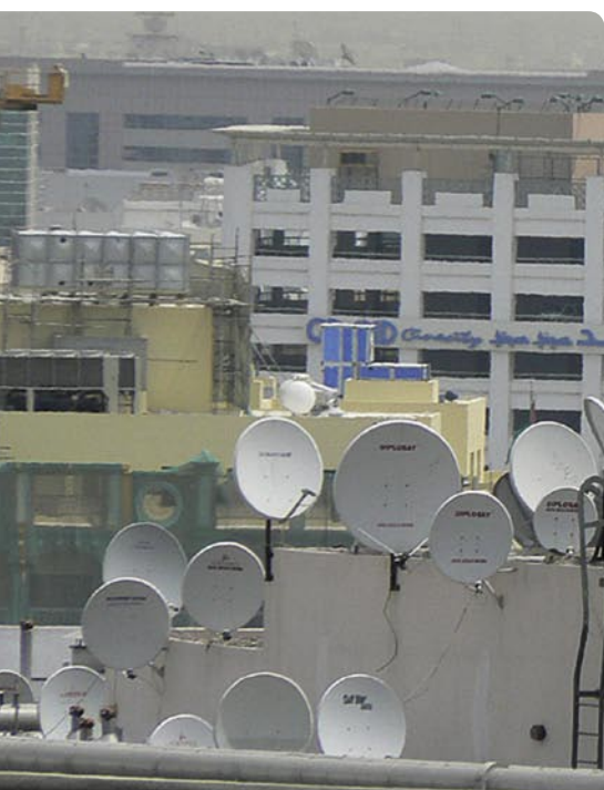
Everyone squeeze together for the picture: numerous dishes installed one right next to the other. Don't worry, there's still room for a few more.
