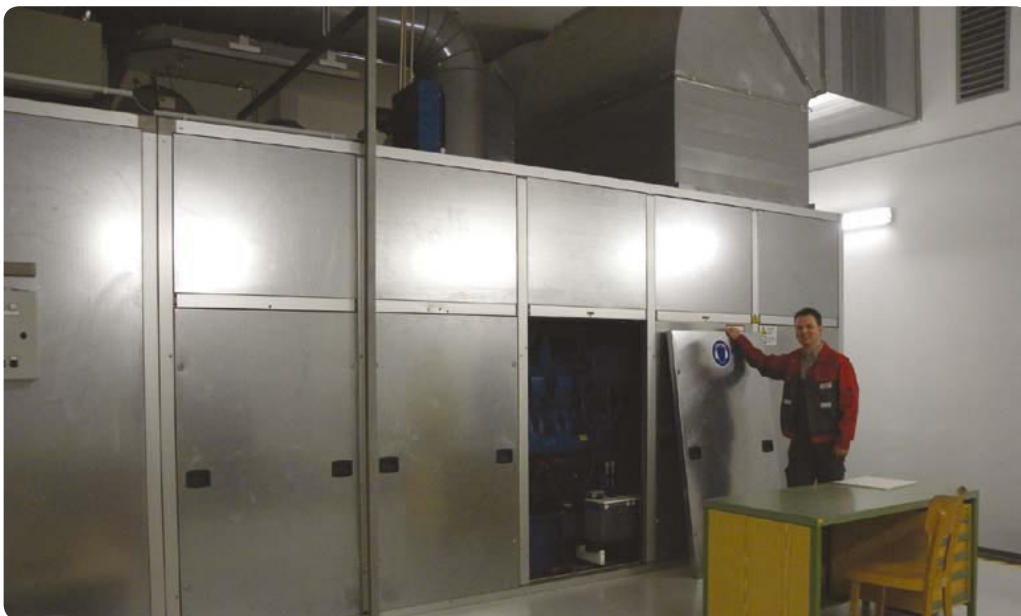
■ The Usingen earth station is a professional operation which means that failures of the public power grid must be compensated. Seen here is one of two diesel generators which are capable of providing enough power for all transmission components. Approximately once a year there is a real power failure (if a power line is cut during road works, for example) and in such a case the back-up systems starts automatically. "About twice a year we experience scheduled power outages which are necessary for maintenance or repair of the grid, for instance," the responsible technician explains. "Apart from that, we let the diesel generators run at capacity for a certain period of time every three months to make sure the engines stay operational at all times." Whenever this is done any excess power is even fed back into the public grid. "We have enough diesel available to run our generators for four weeks in a row," the technician emphasises that the Usingen earth station is self-sufficient for prolonged periods.
