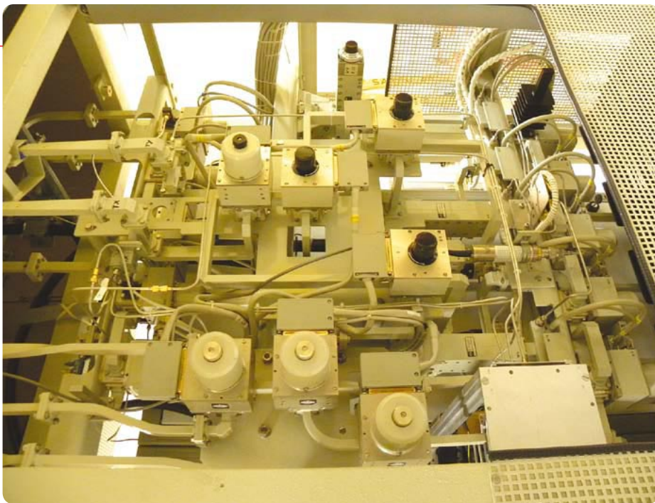
■ Inside one of the huge antennas: hollow conductors are used to guide and switch satellite signals.
